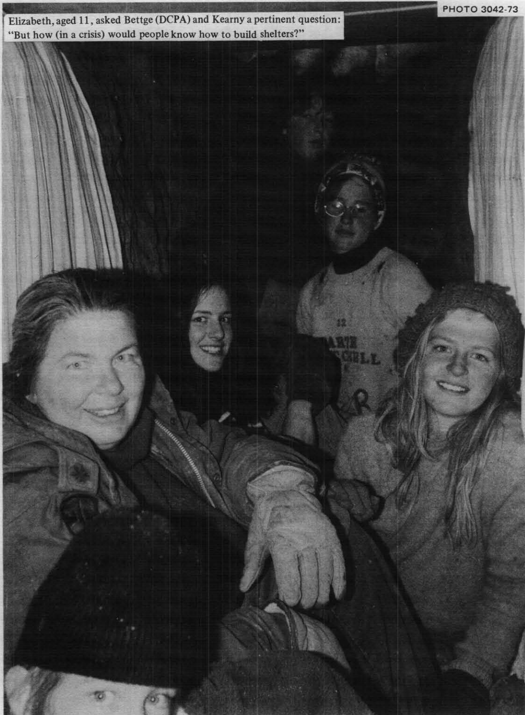
Fig. 2.12. Inside their completed Door-Covered Trench Shelter, and all pepped up by their success in finishing an unexpectedly hard job. They completed their shelter at 3:50 PM on November 25, about 34 hours after first receiving the instructions on November 24.
